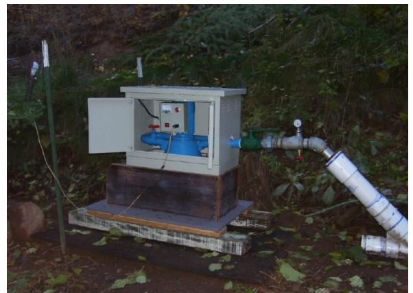
Figure 10: A Realtime Completed Installation of a 5kW Hydro Power System
